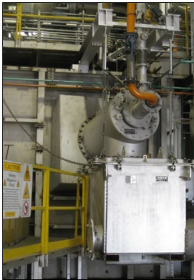
Figure 5. Close-up of one of the four Bloom regenerative burners.
