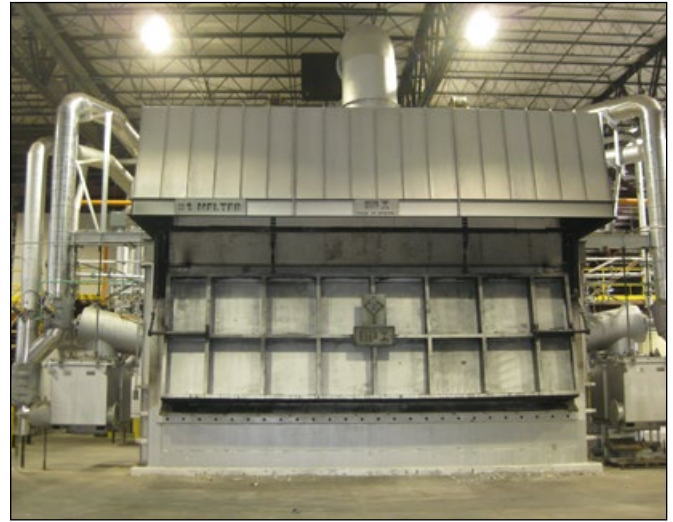
Figure 3. New 220,000 lb G&P furnace.
