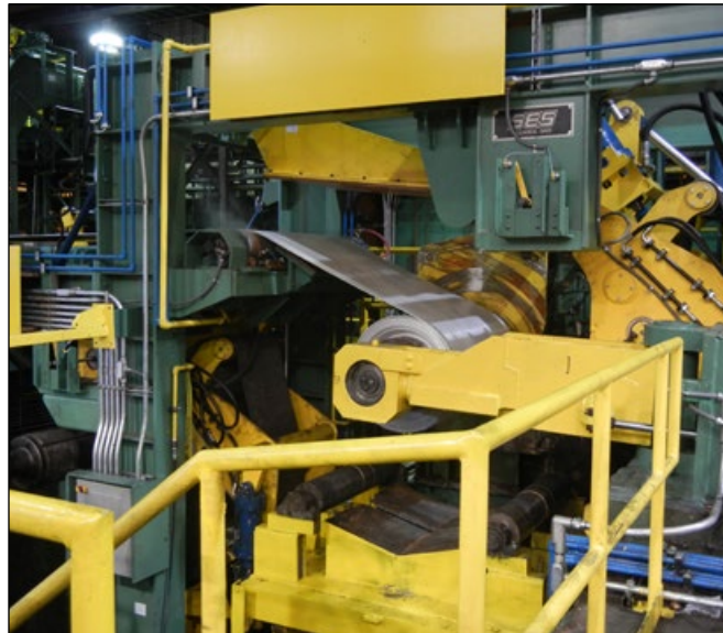
Figure 6. The upgraded aluminum mill shown with new belt wrappers.
